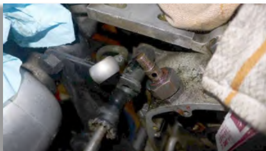
Figure 23: Disconnected vent pipe at the timing cover.
