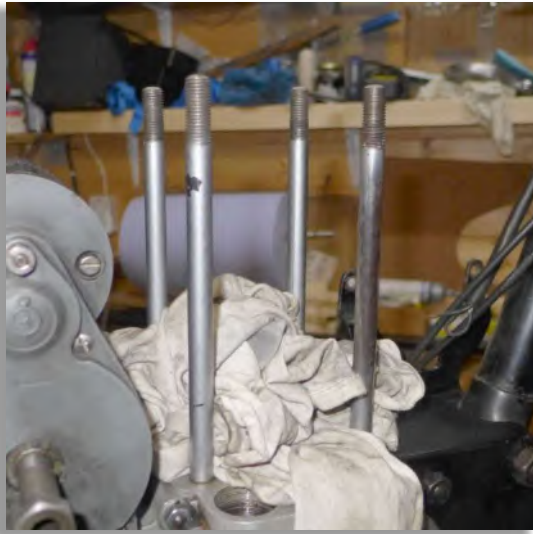
Figure 77: The chrome surface of the front right cylinder stud in poor condition.
